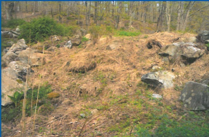
Indications of overtopping at right of spillway
