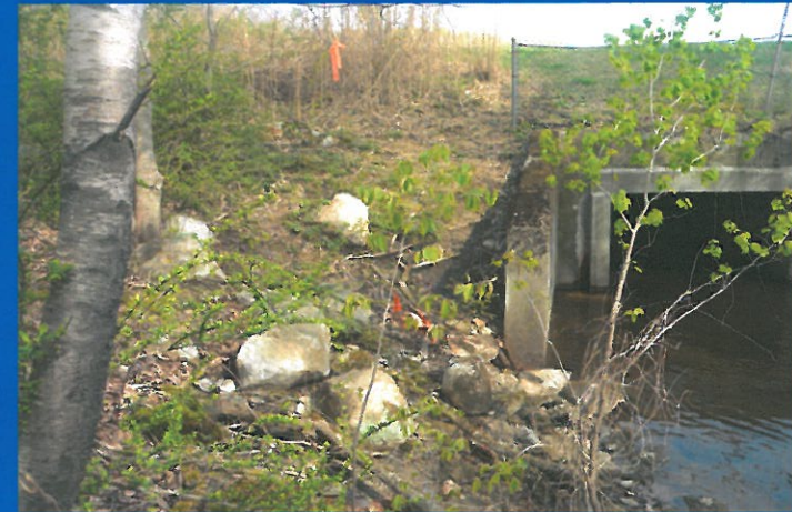
Erosion at spillway culvert outlet walls
